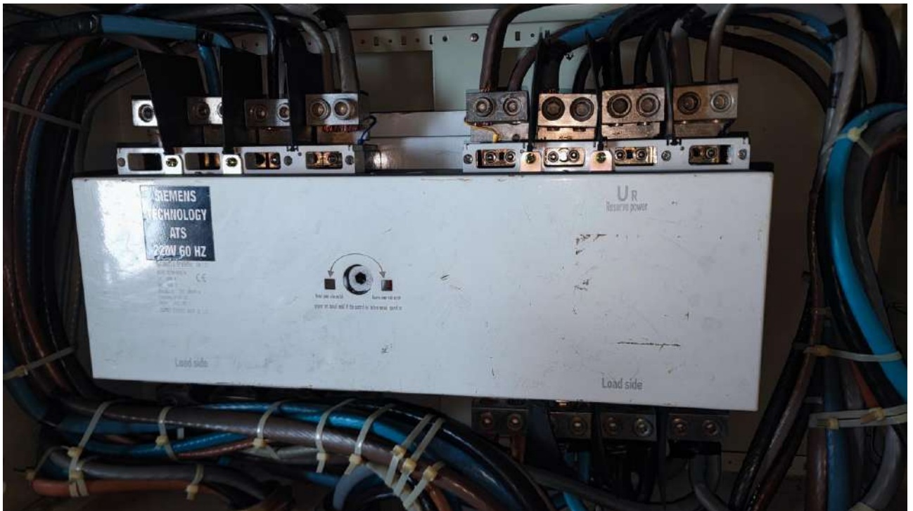
Automatic Transfer Switch
