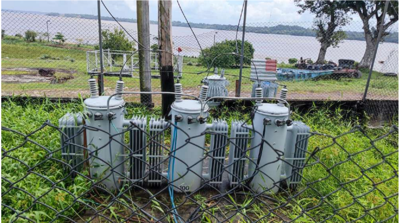
Existing Step-Up Transformers
